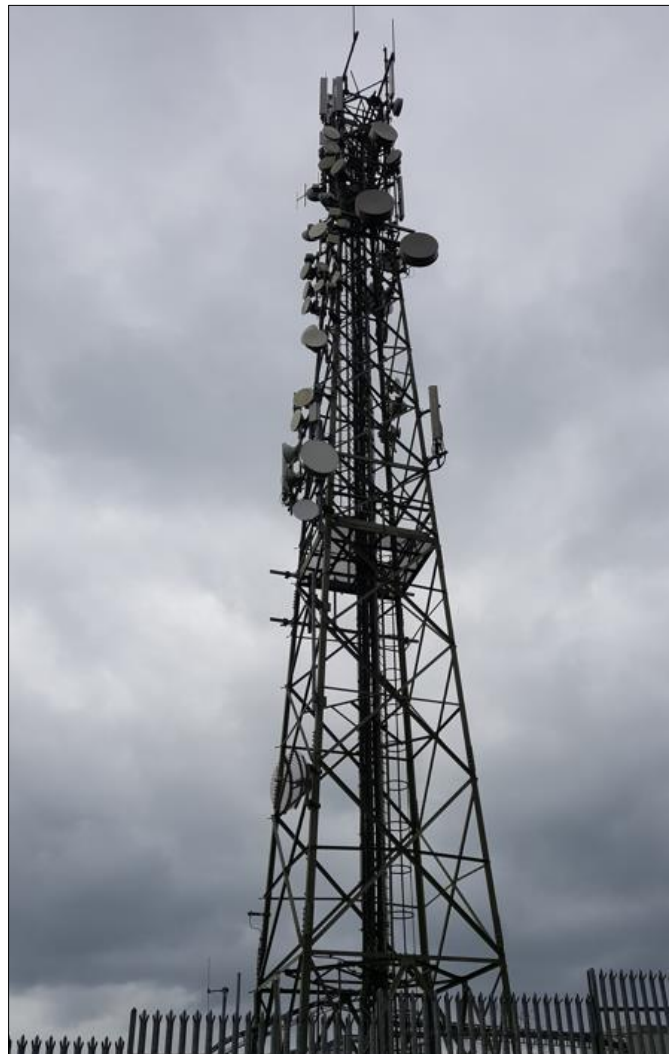
Figure 2. Telecoms Mast at Laghtseefin
