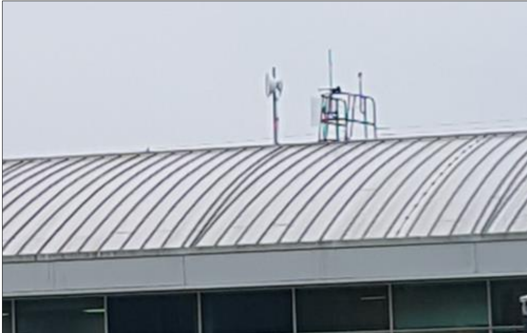
Figure 7. Telecoms Mast-structure at Amneal
