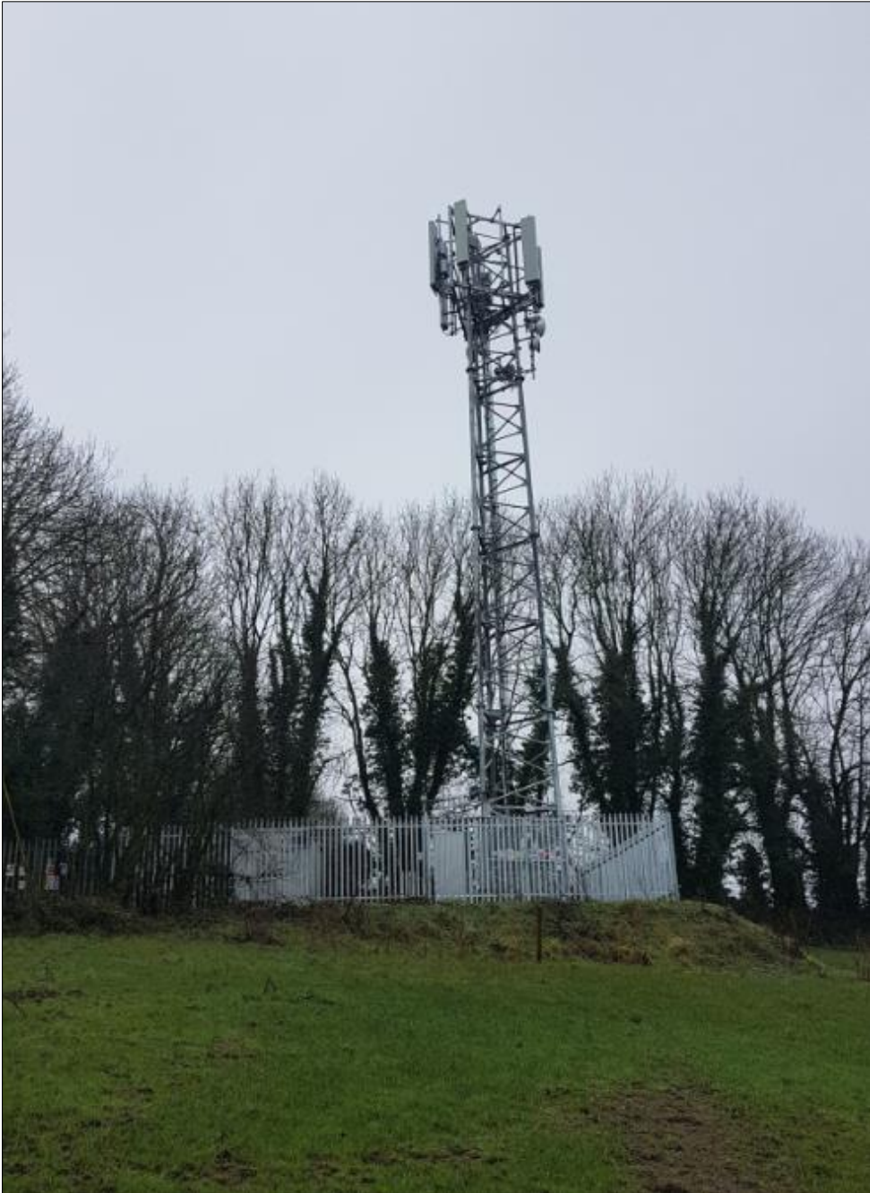
Figure 9. Telecoms Mast at Clonouty
